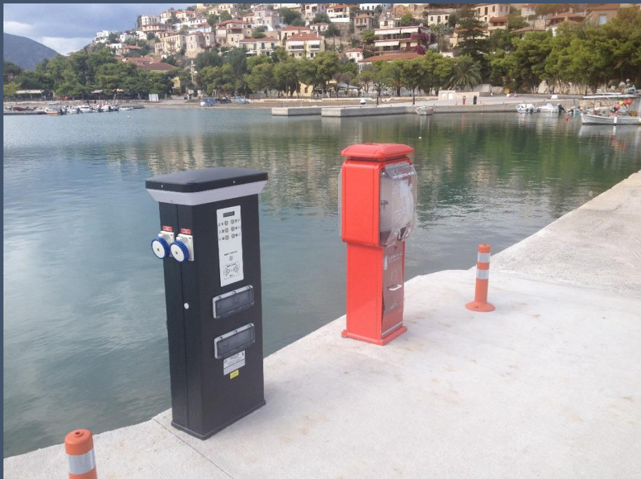
Electricity – watering pillar + fire fighting pillar
